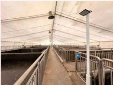
Super Factory coating wastewater treatment
