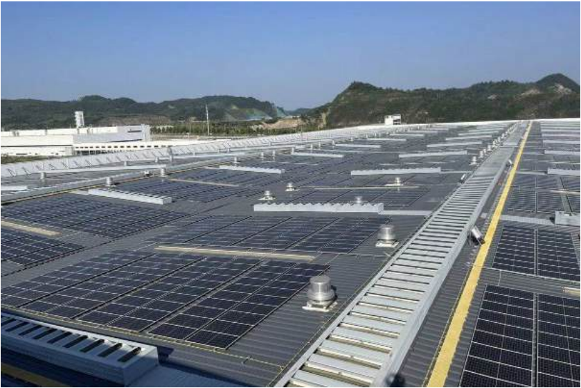
Rooftop photovoltaic devices installed for warehouses
